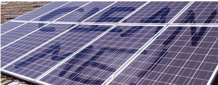
Figure 19. Soiling on PV modules
