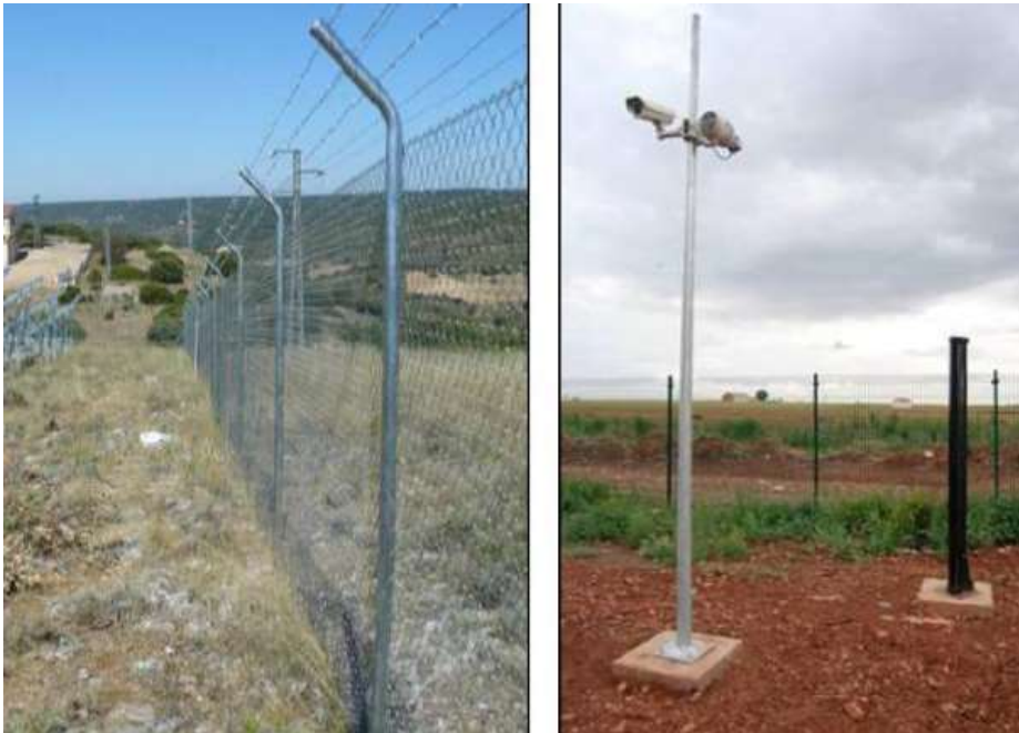
Figure 75. Example of Security Systems used in PV power plants
