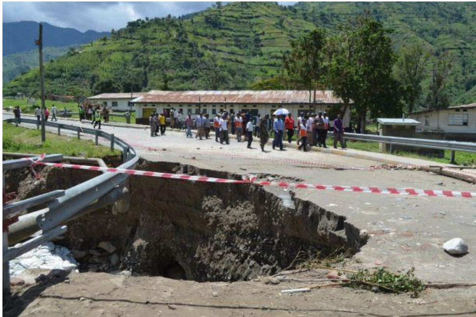
Figure 1: Flood damaged to a paved road.
