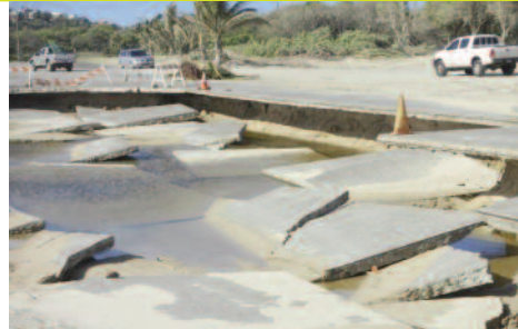
Figure 2: Destruction to the Vieux Fort Highway caused by seawater inundation. Without action more intense storms brought on by climate change will continue to cause costly damage to infrastructure. (Source SLNT)
