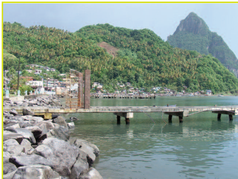
Figure 3: Coastal protection measures are in place to try to protect the coastal village of Soufriere from storm surges and sea level rise. (Source CANARI)
