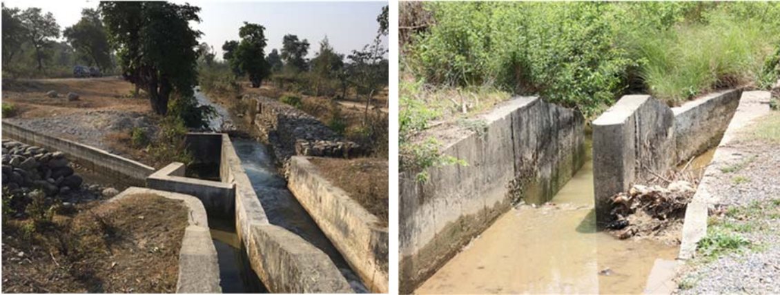
Figure 19: Singhghat canal structures
