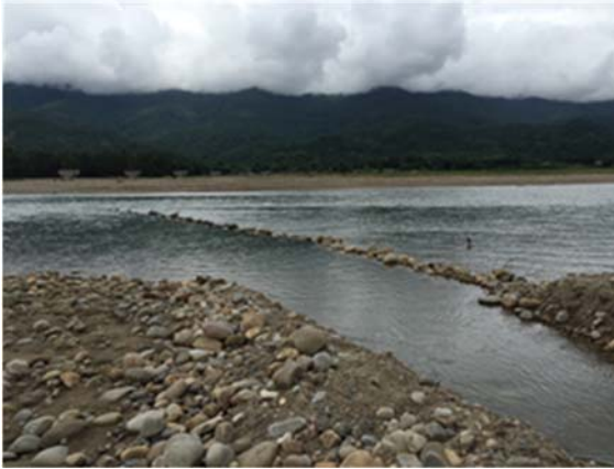
Figure 6: Nepane Irrigation Intake
