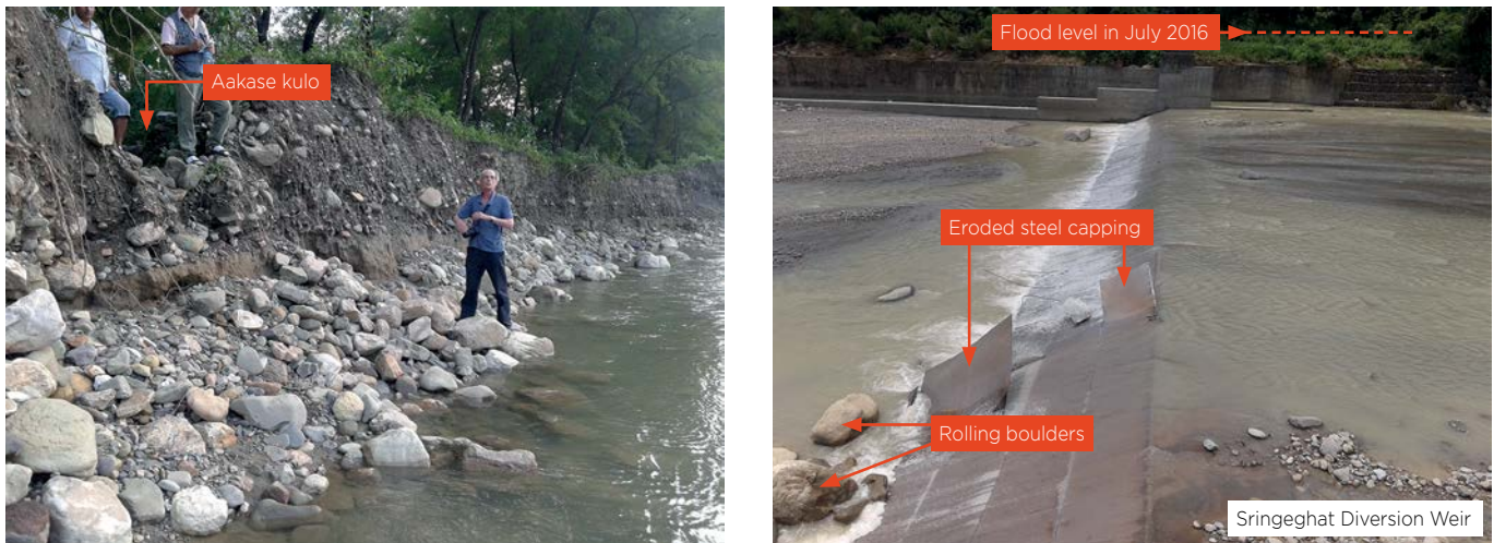
Figure 4.4. Flood damage of intake and weir
